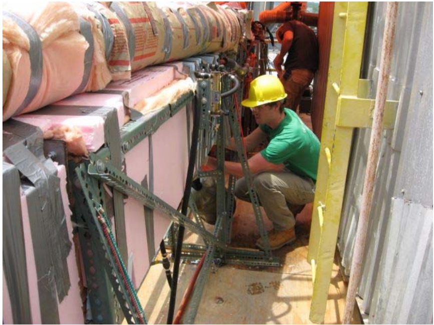
Measurements Being Made with Condensing Heat Exchanger Apparatus During Slip Steam Field Test.
